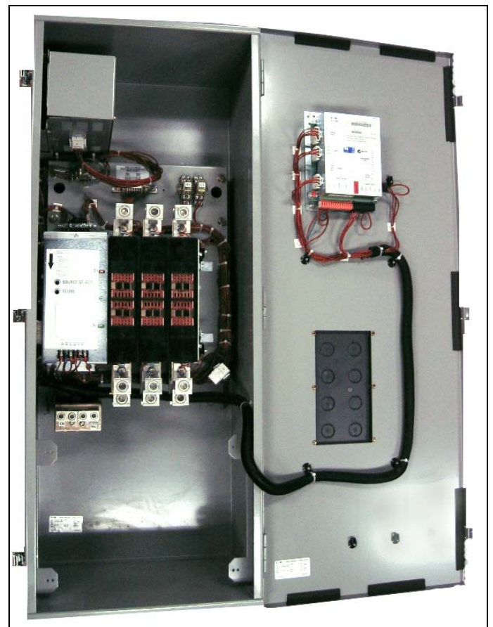
Figure 10. Typical (40A-400A) Contactor Based ATS Equipment (Door Open).
